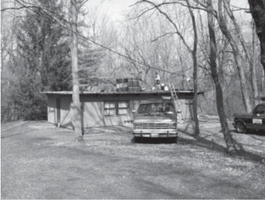
Both the Hickory and Sycamore dorms recently got new roofs, thanks to the GHA.
